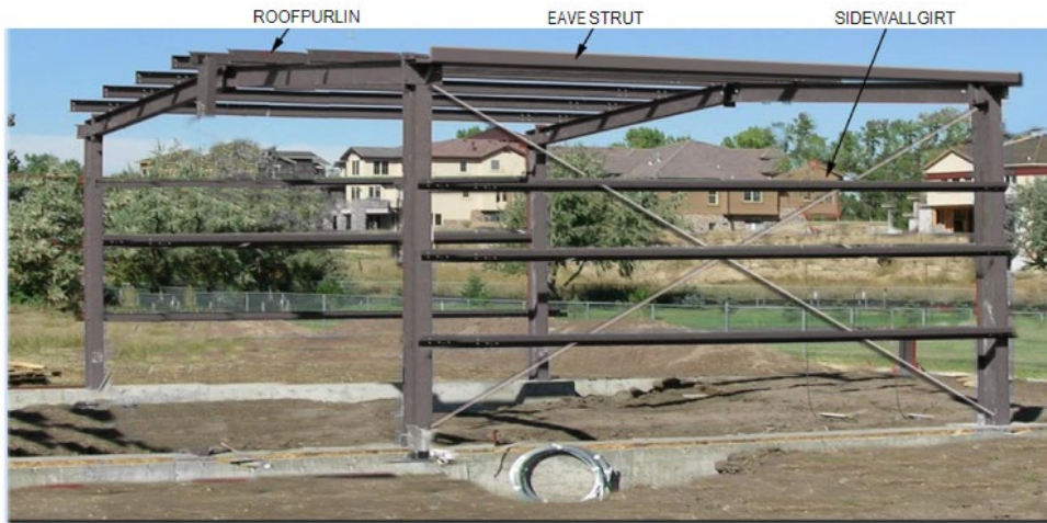
Illustration above shows a bay under construction. The cable bracing on the sidewall has been highlighted to better show the detail.
